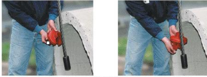
Drop pipe carrier lifting sling through hole in pipe. Align and insert "Tea Cup" pipe carrier into lifting sling.
